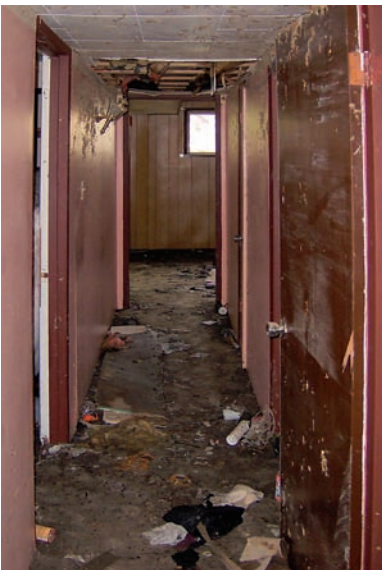
Finished basements experience far greater damages than unfinished basements when the basement floods.
