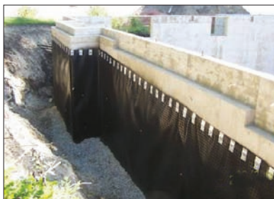
A gap around the basement wall in a home that is under construction.
