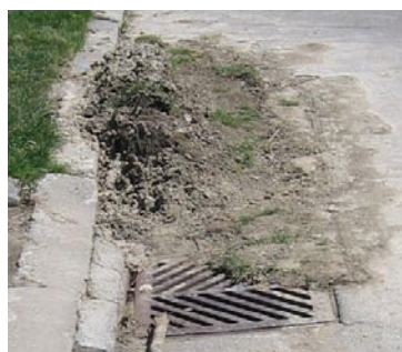
Storm sewer grates that are free of debris are better able to handle stormwater flows and can reduce overland flooding.
