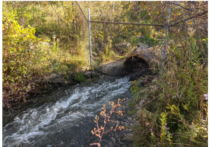
PHOTO 2: Culvert going under New Lakeshore Road at Stelco Creek. Photo was taken facing south.
